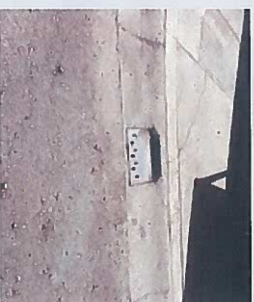
SETTLEMENT DUE TO FILL PLACEMENT
